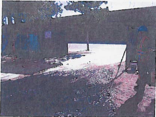
Exhibit 4: Entrance to larger work area showing 3/4" gravel, a shaker plate, and minor tracking where vehicles by-passed the shaker grate to the right.
